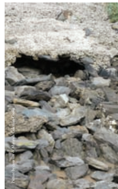
TIDES ERODE BENEATH MODERN CONCRETE REPAIRS
